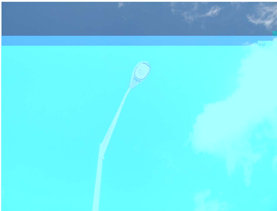
Example of Cobra Head LED Retrofit Unit (Holly Drive and West Entrance to CPT)
