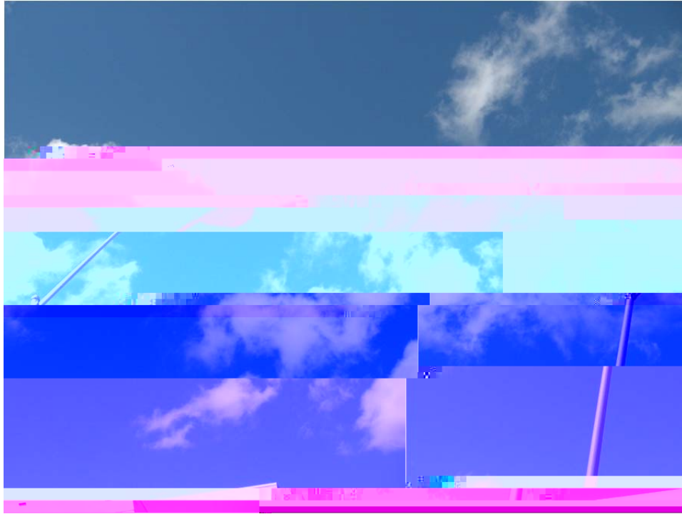
Typical Campus Cobra Head, High Pressure Sodium, Light Fixture
